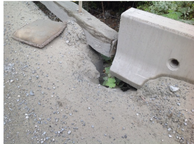
fill erosion left upstream approach
