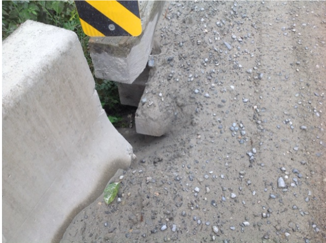
fill erosion left downstream
